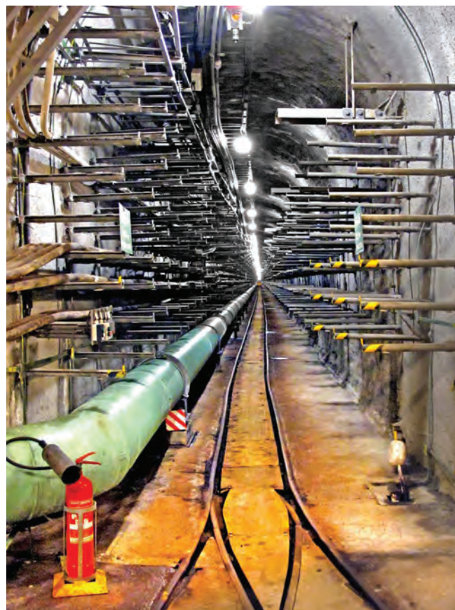
Racks carry a myriad of services within the Kolektory centre and strolled back to our starting point through the morning tourists and residents.
